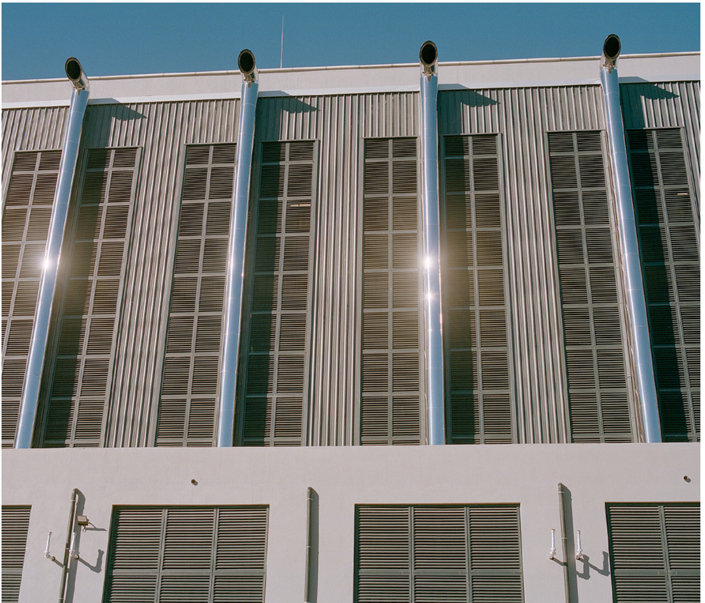
Large aluminium vents protrude from the Teraco building, likely used to maintain steady airflow and control temperature.
